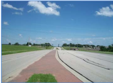
Improvements at US-40/K-10 Interchange including signalization at the ramps and along US-40 east of K-10 would be short term needs. (Existing shown)
