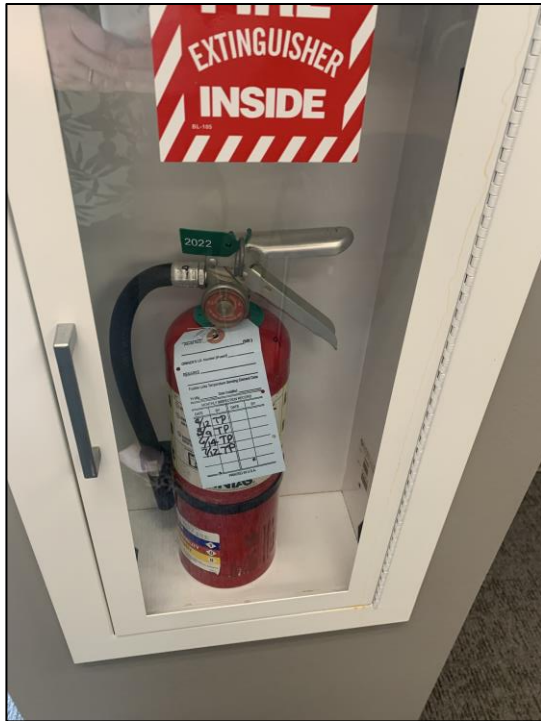
Figure 6: Fire Extinguisher Examples (Photos: TranSystems)
