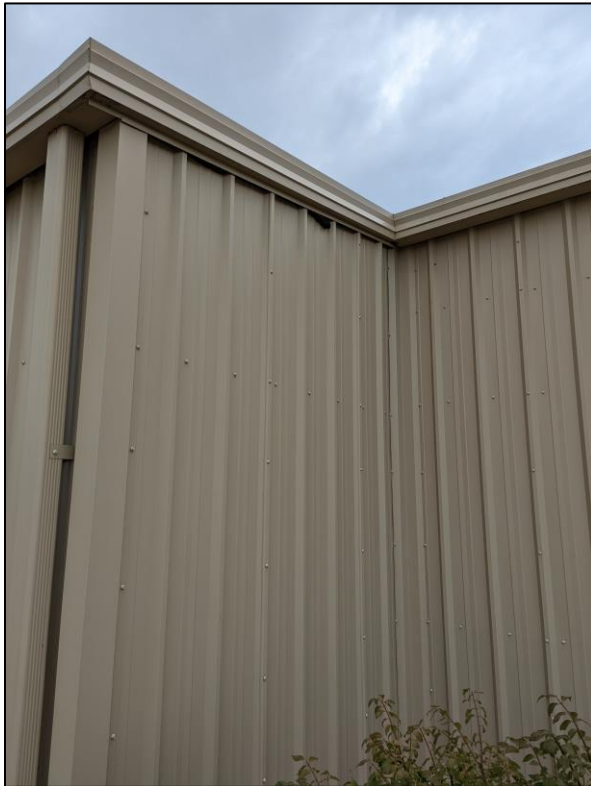
Figure 2: Exposed Insulation Example (Southwest Exterior) (Photo: TranSystems)
