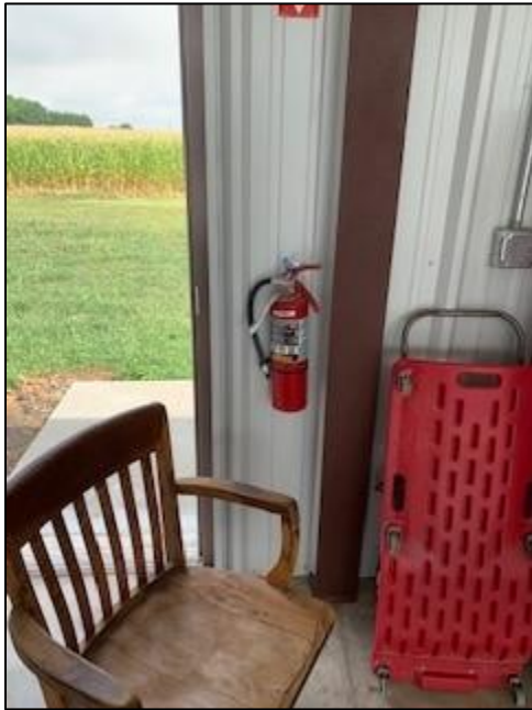
Figure 5 & 6: Fire Extinguisher Locations (Photos: KDOT)
