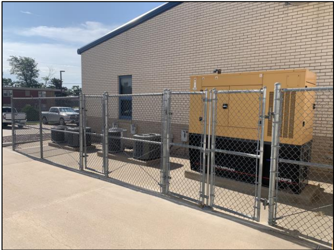
Figures 5 & 6: HVAC and Extinguisher Examples (Photos: TranSystems)
