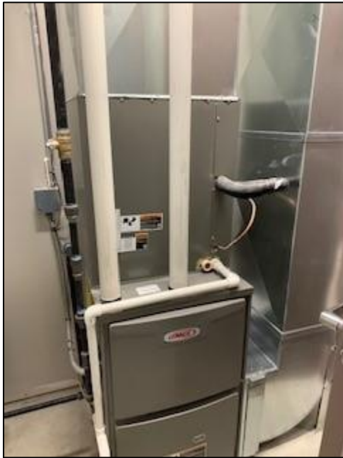
Figure 4: Facility HVAC (Photo: KDOT)
