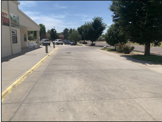
Figures 8 – 9: Concrete Wear Examples Surrounding Facility (Photos: TranSystems)
