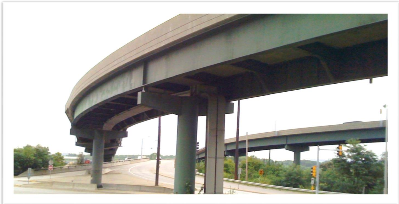
The girders and piers on this ramp structure in Wyandotte County are Fracture Critical Members.
