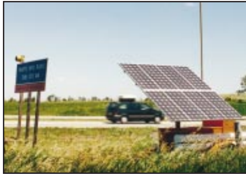
The highway advisory radio and flashing light are powered by a portable array of photovoltaic cells.
