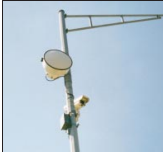
Freeway surveillance camera and antenna at intersection
