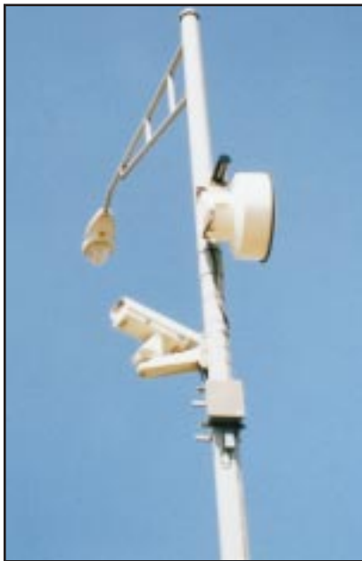
Intersection signal pre-emption device
