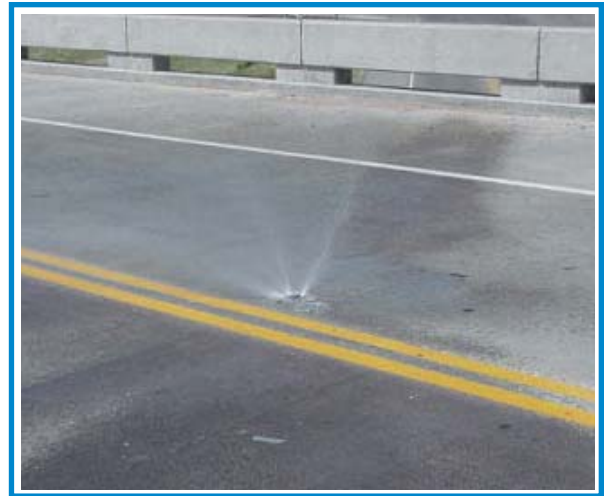
An example of a spray nozzle spraying chemical onto the pavement surface.
