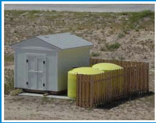
The shed that houses the pump and controls and the storage tanks for the anti-icing system.
