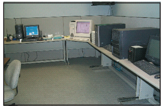
Traffic Operation Control Room
