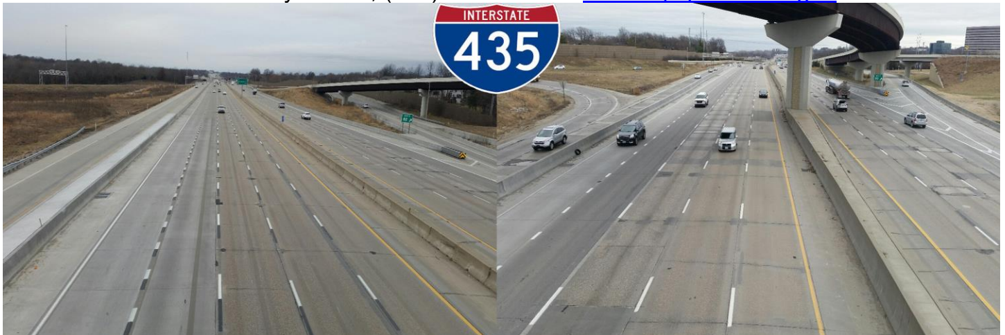
A 'before look' at existing deteriorating concrete pavement along this stretch of I-435.
