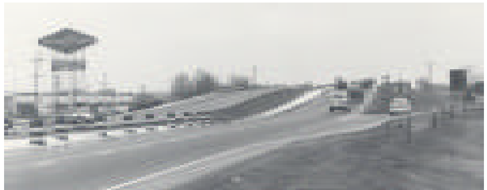
Rehabilitation work will take place on the eastbound US-24 bridge over Goodyear Road with traffic reduced to one lane in each direction.
