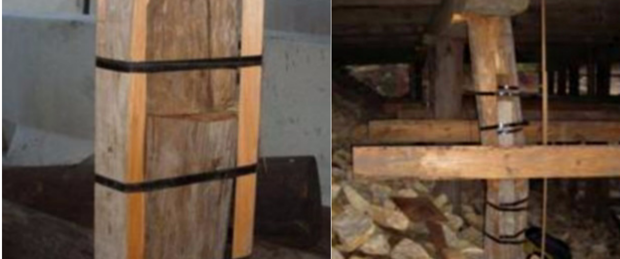
Figure 19: Potentially Dangerous Column Splice Details
