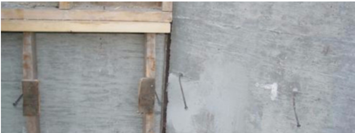
Figure 10: Remaining Break Off Ties
