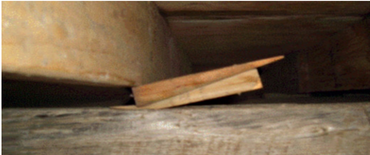
Figure 20: Incorrect Shim Placement
