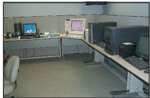
Traffic Operation Control Room
