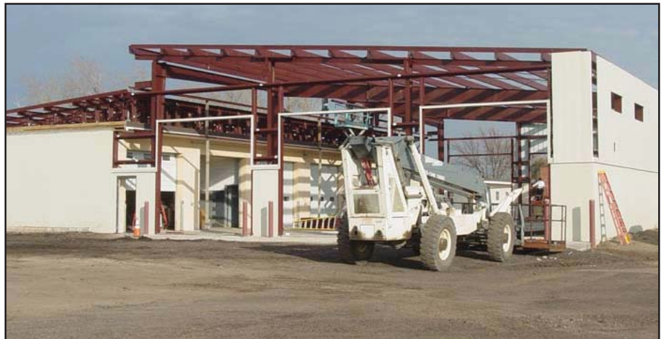
Progress continues on the new 60-foot by 100-foot extension to the Garden City Subarea's truck bay.
