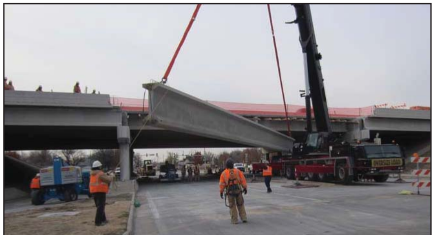
Above and left, the new beam is installed on the U.S. 50/400 bridge.
