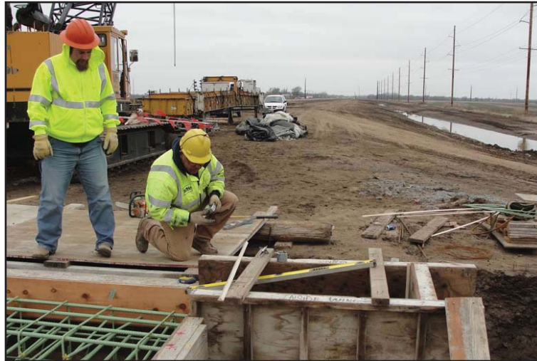
Eric Smith, newly-promoted Engineering Technician (ET) Senior, left, inspects a bridge being constructed on the U.S. 50 four-lane expansion project in Hutchinson.
