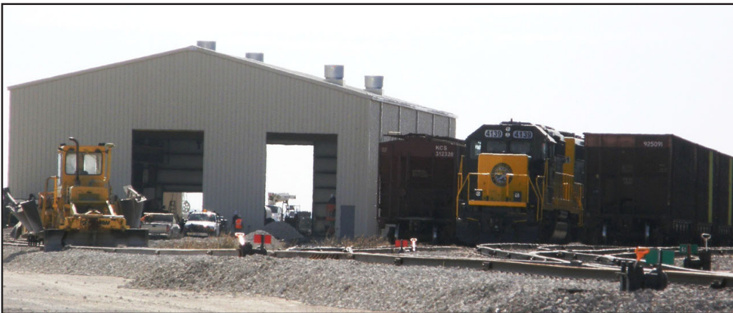
Work continues on construction of a new mechanical shop at the South Kansas & Oklahoma Railroad yard north of Cherryvale.
