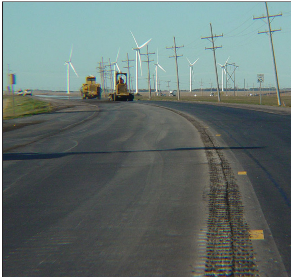
A crew from Dustrol, Inc., grinds in center line rumble strips on U.S. 50/56 near Spearville in Ford County. The center line rumble strips were added as part of a resurfacing project.
