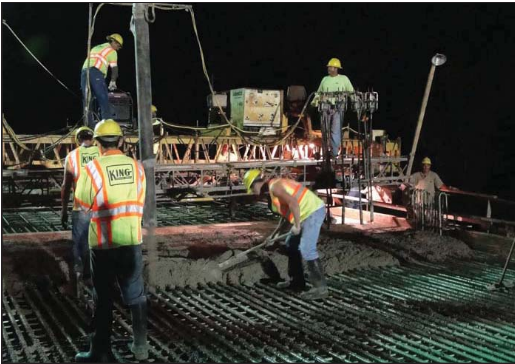
At left, King Construction does a bridge pour at night for a new K-14/K-96 bridge south of Lyons.
