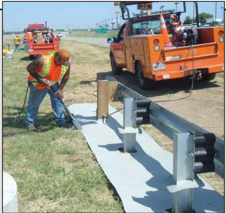
Equipment Operator Chris Riggs installs a roadside weed barrier along I-135 in Wichita.
