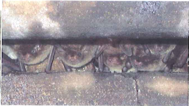
Photo 2: Visible bats within an expansion joint
