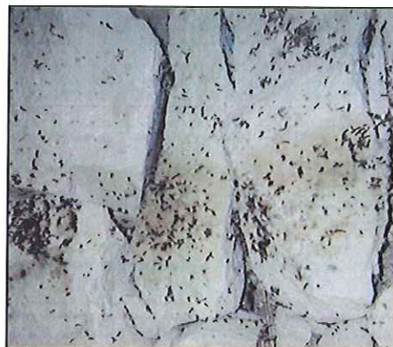
Photo 6: Bat Guano on Rip Rap
