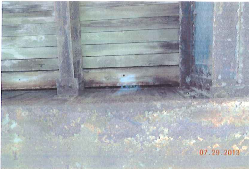
Photo 14: NLEBs Roosting Under a Timber Decked Bridge
