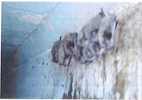
Photo 1: Bats hanging from cracks along Support beams
