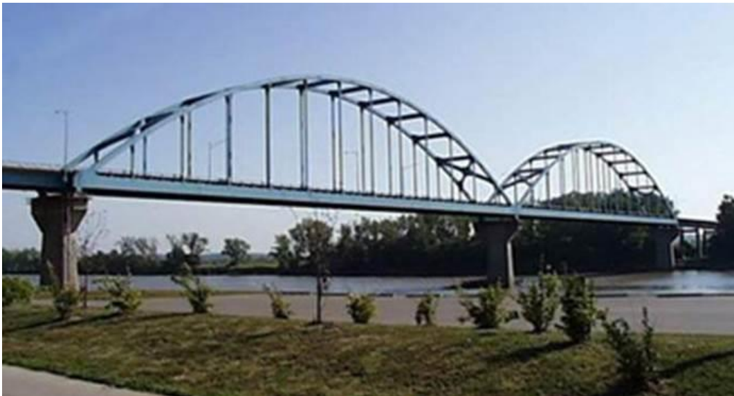
A look at the existing Route 92 Centennial Bridge spanning the Missouri River.
