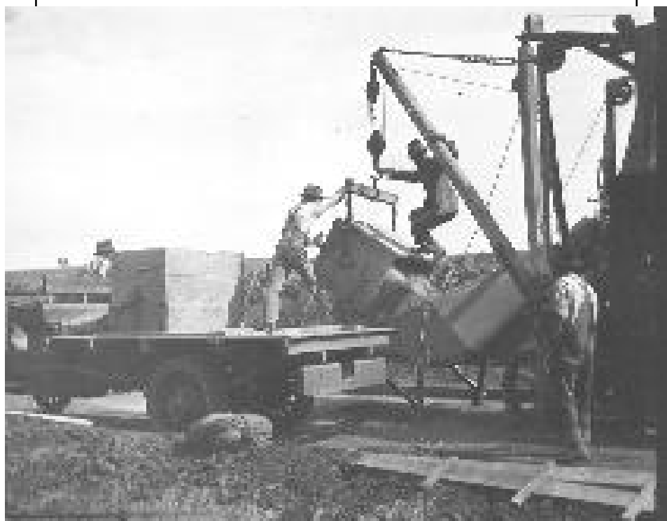
Workers build a new roadway in Mitchell County during construction activity in July of 1919.
