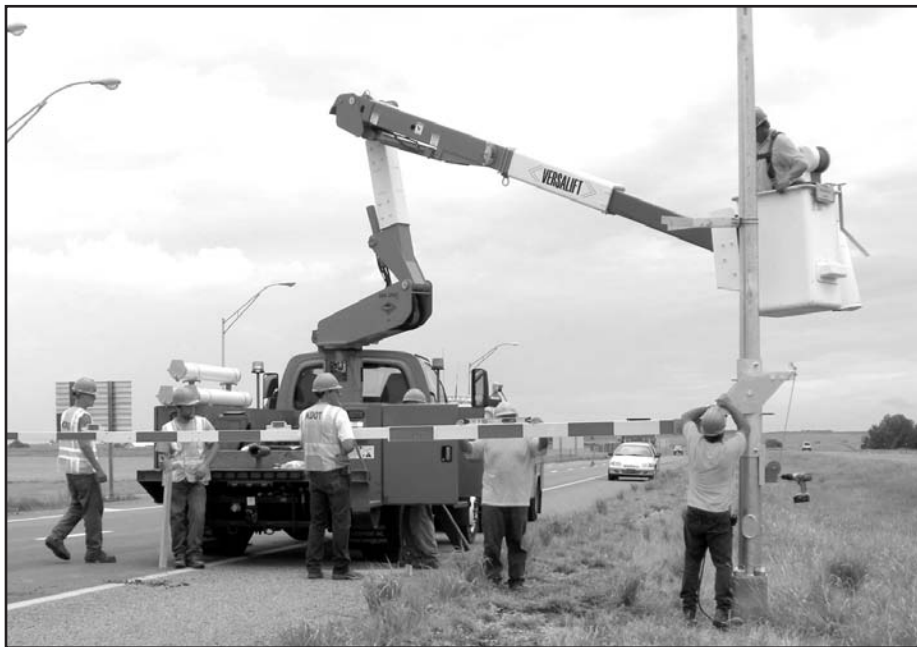
A crew of KDOT employees from different offices in District Three install snow gates along I-70. Photo by Kristen Brands
