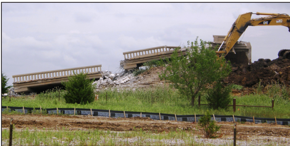
The ATSF Railroad bridge at Welda is torn down. Photo by Priscilla Petersen
