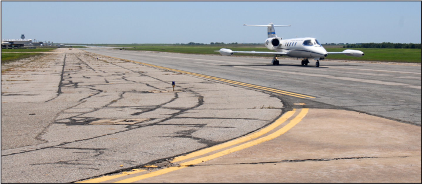
A project at the Salina Municipal Airport will rehabilitate two of the taxiways. Airports across the state will receive various improvement projects. Photo by Kurt Weaverling
