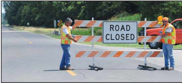
Troy Subarea employees Pat Jasper, Equipment Operator Senior, and Jim Clary, Subarea Supervisor, close a portion of K-7 due to flooding.
