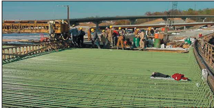
Work to pour the concrete deck on the northbound I-635 bridge over the railroad yard takes place in early November.
