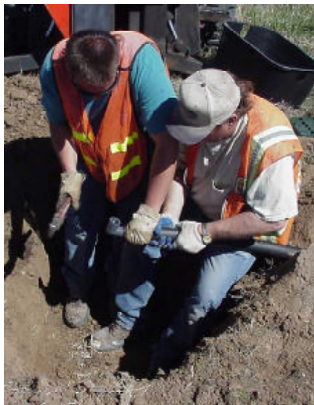
Last summer, District Six employees Andy Barton and Jimmy Gilbert install the pipe for the fixed anti-icing system on the US-50/83 and K-156 interchange.
