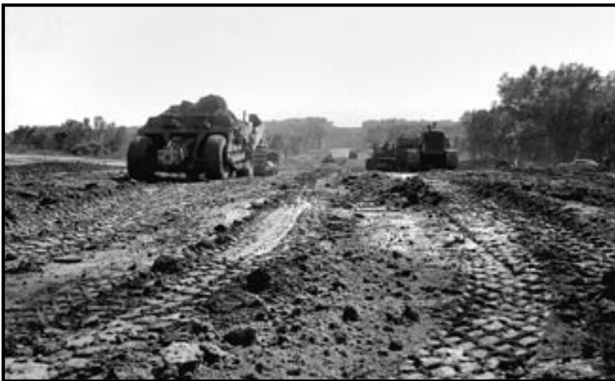
Roadway is cleared for the construction of US-75 north of Holton in October of 1957.
