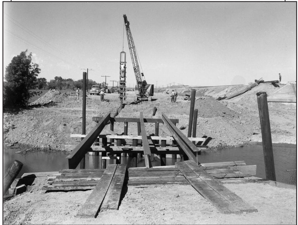
Replacement of the K-383 bridge at Clayton in Norton County during the summer of 1953.
