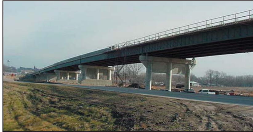
On the west side of Marysville, a US-36 bridge is being constructed over the Big Blue River, the Union Pacific Railroad and a new levee. Photos Courtesy Wamego Area Office.
