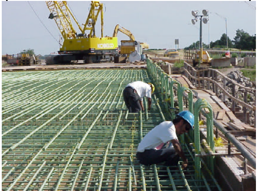
This I-135 bridge south of Mentor Road is getting ready for the deck to be placed.
