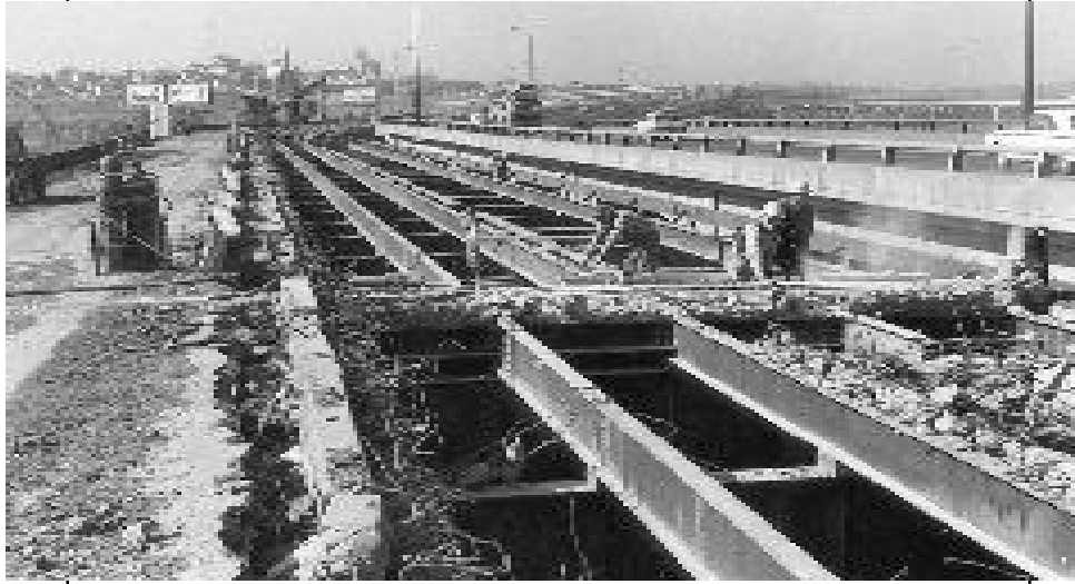
The old deck of the Intercity Viaduct in Kansas City is removed during a bridge rehabilitation project in February of 1963.
