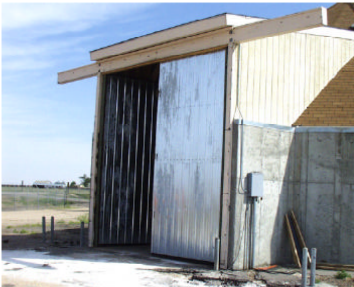
The idea to install new metal doors that swing inward on the salt dome in Lakin proved to be very effective.
