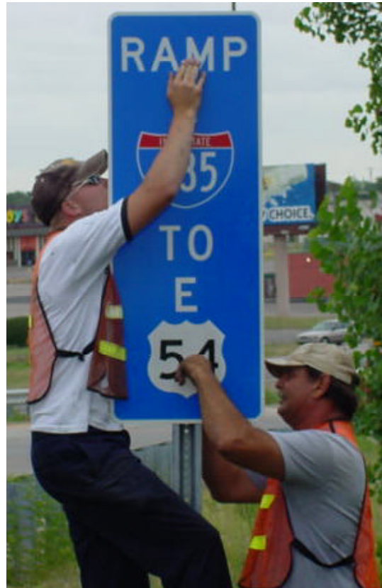
Heath Bissel, left, and Sam Juul, Paul J. Fulsom Construction Company employees, install new route reference markers along US-54 in Wichita.
