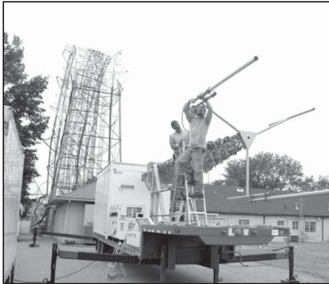
KDOT employees Bryan Hardwick (left) and Jeremy Belleau install the antennas on the temporary tower which is located north of the damaged communications tower (in the background) that fell during a storm on June 12.
