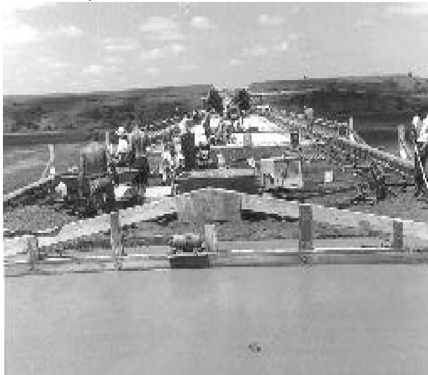
Concrete was laid for new Interstate 70 in northeast Kansas during construction activity in June of 1962.
