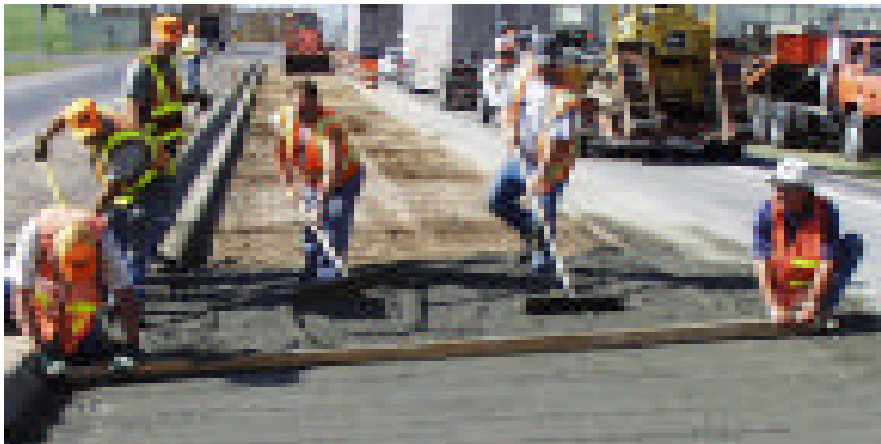
Jack Immroth (far left) and Gerry Pearson (far right) use a two-by-four to level off the concrete, as Kenny Gibbons, Jesse Casanova, Tim Deaver, and Jimmy Gilbert work it with shovels and rakes.
