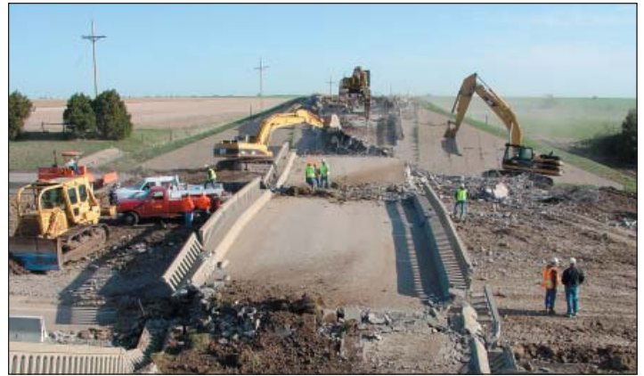
It took about 6 1/2 hours to remove the bridge and reopen I-70 in Russell County.
