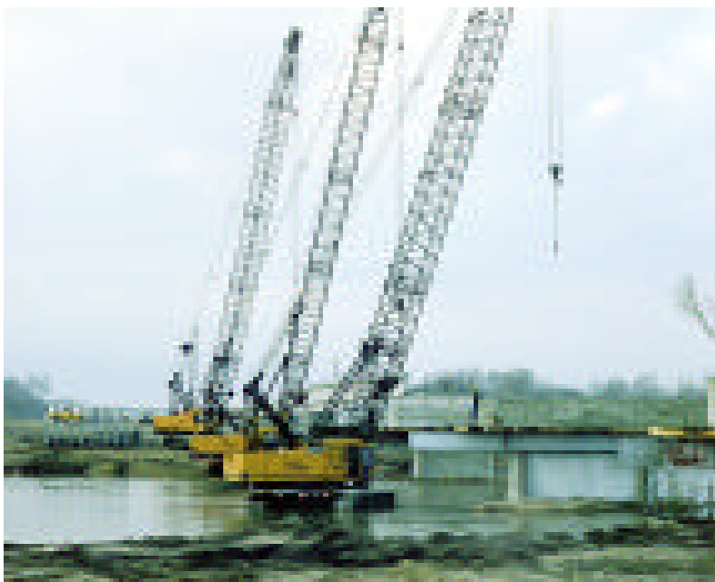
A bridge over the Arkansas River is constructed as part of the $42 million Hutchinson bypass project.
