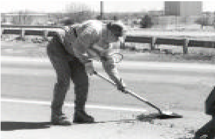
Dale Patterson, Equipment Operator at the Area Four office in Topeka, fills a pothole on US-75.
