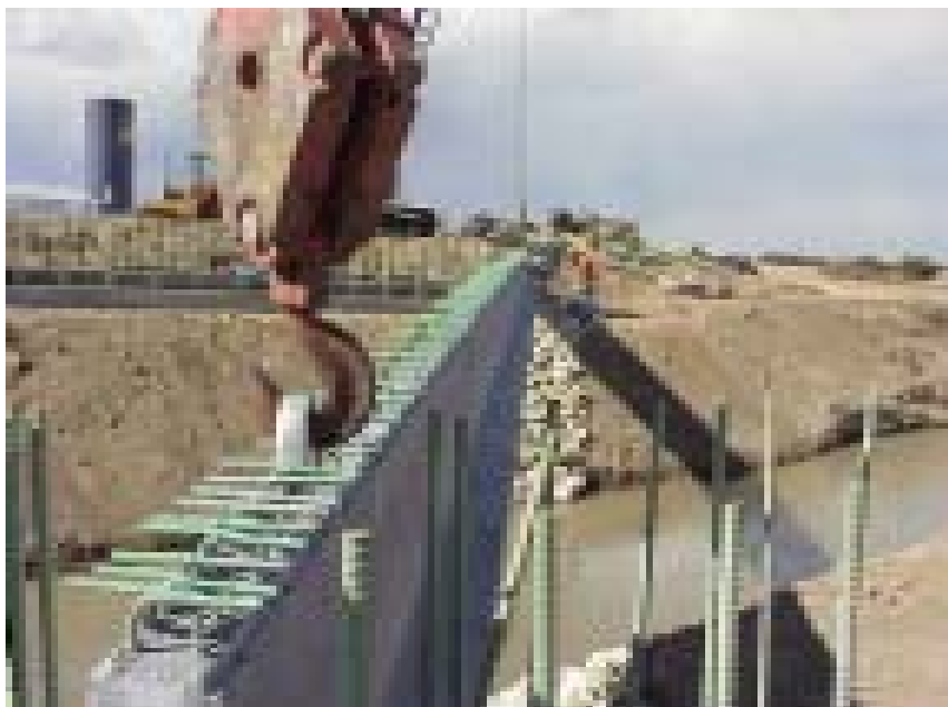
A concrete beam is set in place on K-25 north of Lakin. It is the first bridge project in Kansas to use inverted 'T' prestressed concrete beams.
