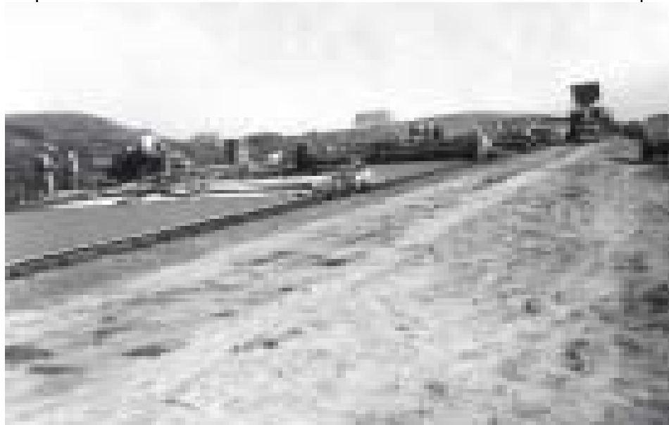
Interstate 70 construction in Kansas was in full swing during this picture taken in October of 1964.
