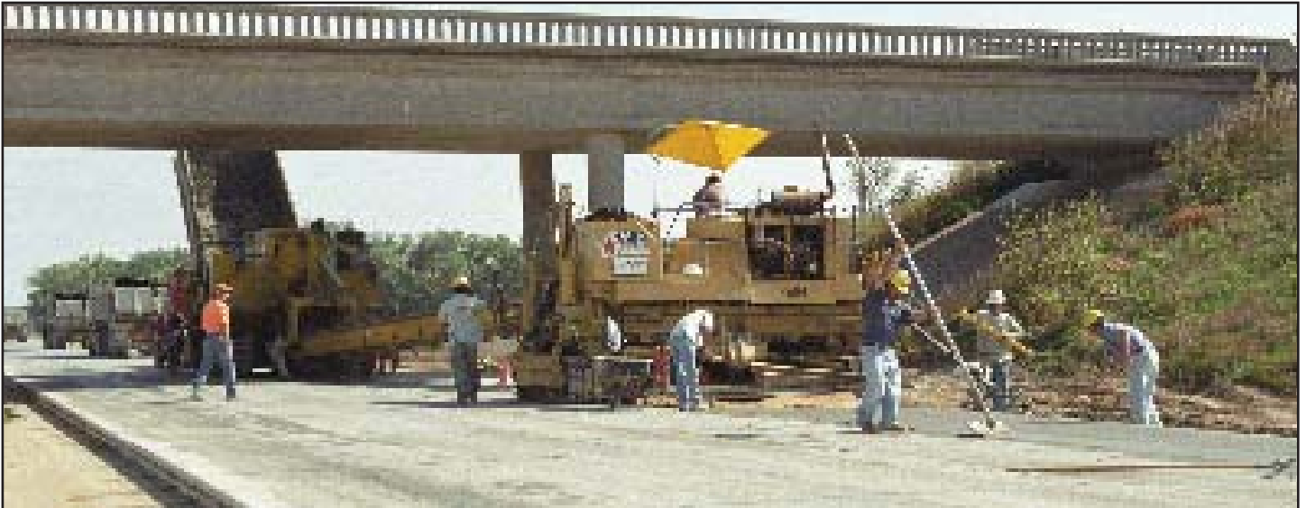
I-70 reconstruction work continues this fall east of Salina. Photo by Kurt Weaverling
