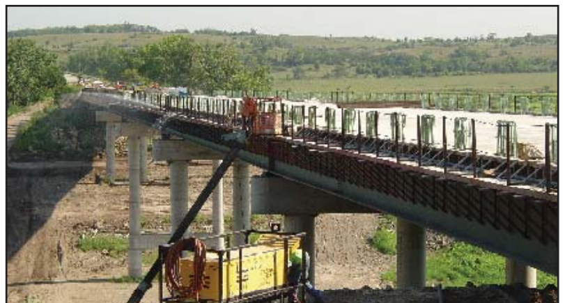
Construction of the new Fancy Creek Bridge is now complete. Photo submitted by District One
