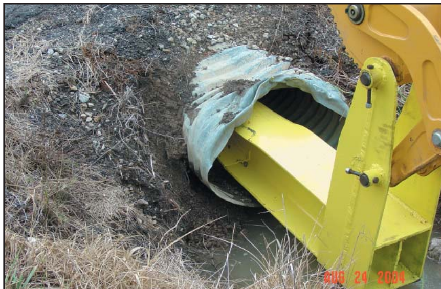
This highly-effective, custom-made culvert end opener was created in the Iola Subarea shop using scrap metal and an expenditure of only $26 for welding.
