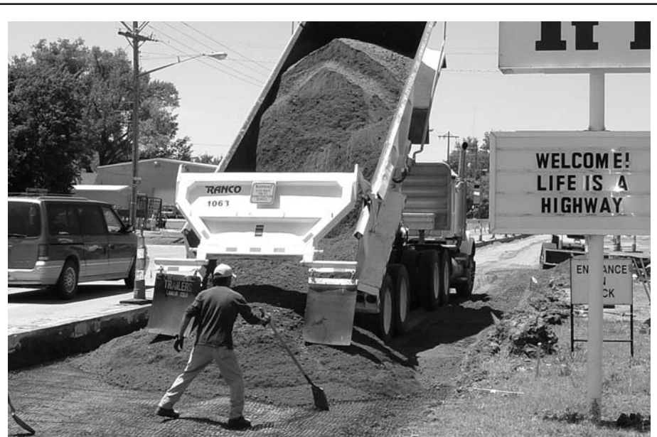
A load of sub-grade mix is placed on U.S. 36 in Atwood as part of a geometric improvement project that is under way from K-25 to Fifth Street. Photo by Kristen Brands
