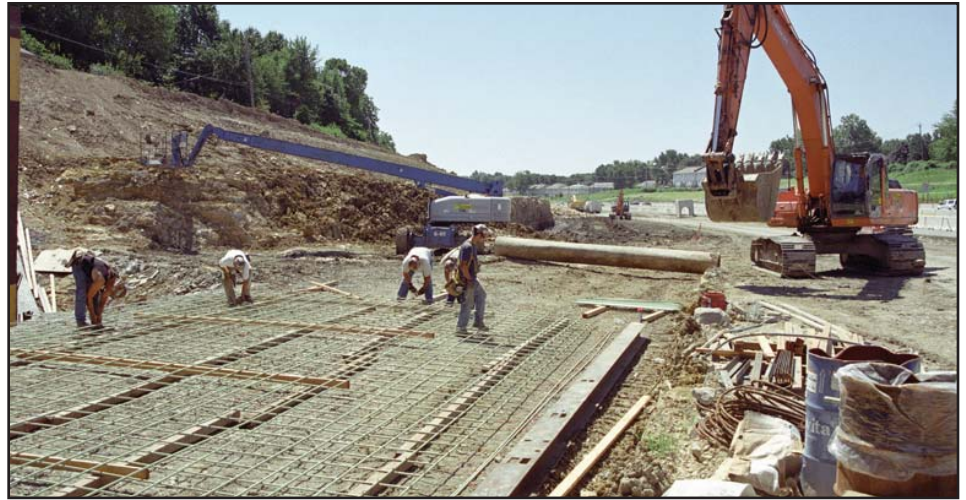
Workers prepare the foundation for a stretch of 91st Street as part of the Recovery Act project taking place along and near U.S. 69. Photo by Kurt Weaverling
