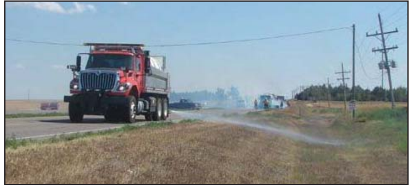
To reduce the risk of fire, a KDOT crew sprays water ahead of work taking place on U.S. 283 in Ford County.
