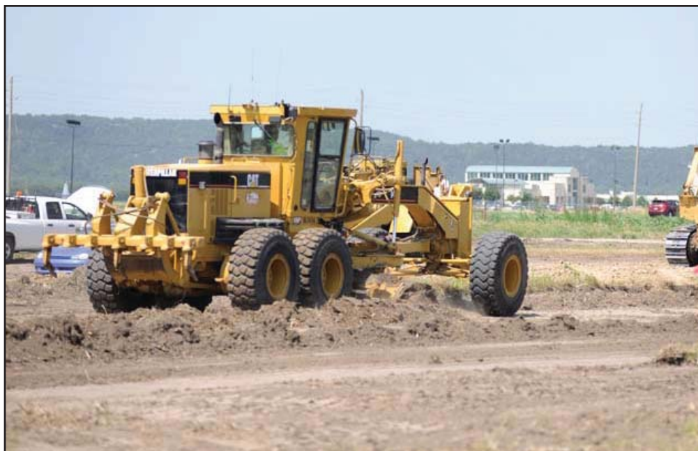
Grading work takes place along part of the K-18 project in Riley County.
