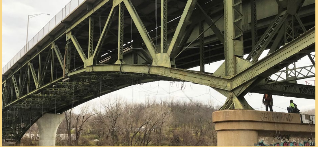
Workers check out the underneath of the 7th St./U.S. 169 bridge as repair work continues. Photo by Joel Smith, District One
