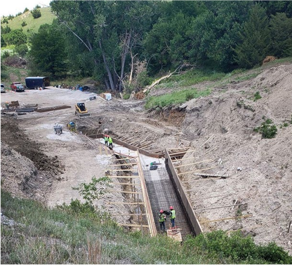
Crews work on prepping the area around a box structure that will be reconstructed as part of the project. The structure is approximately 70 feet underneath the roadway. Photo by Dean Jay, District Three
