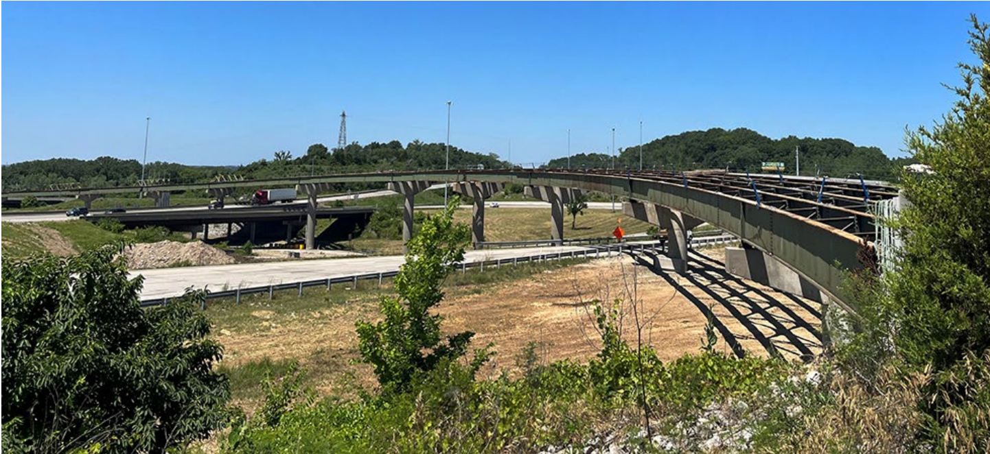
Above is a current view of the flyover ramp with bridge deck removed. Below is a sign showing the location of the project. Photos by Delaney Tholen, District One
