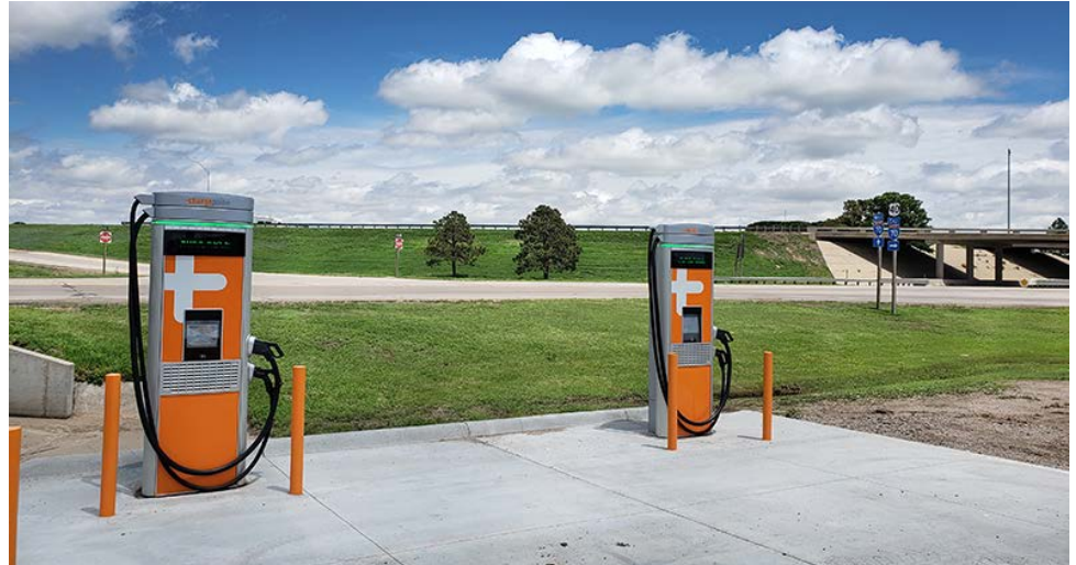
The Oakley EV charging stations opened for service on March 31. The stations are located just off of I-70 at Mitten's Travel Center. Photo by Lisa Mussman, District Three
