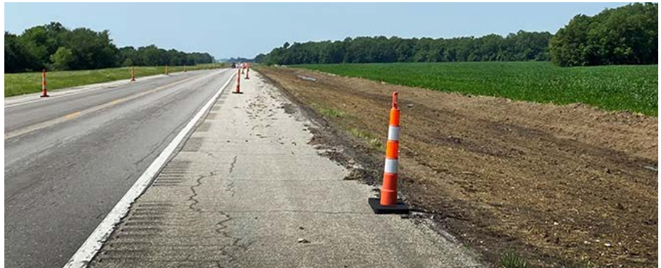
Grading is underway on the U.S. 169 passing lane project south of Thayer.
