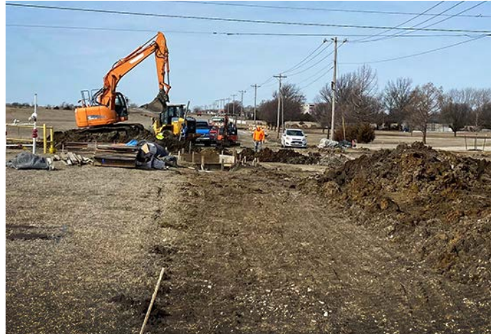
Work is underway at the intersection of Plummer Avenue and 21st Street in Chanute.
