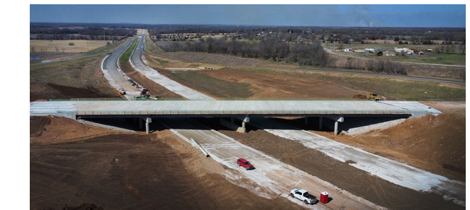
Work is progressing toward an early summer finish on the T-WORKS U.S. 166 realignment and expansion project in the southeast corner of the state. Photos by Chris Ziegler, Pittsburg
