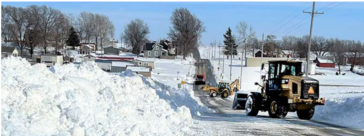
Digging out Crews from Area One work to remove snow from K-20 in Doniphan County. Around 8 inches of snow fell in the area from the two weather systems. Photo courtesy of Area One
