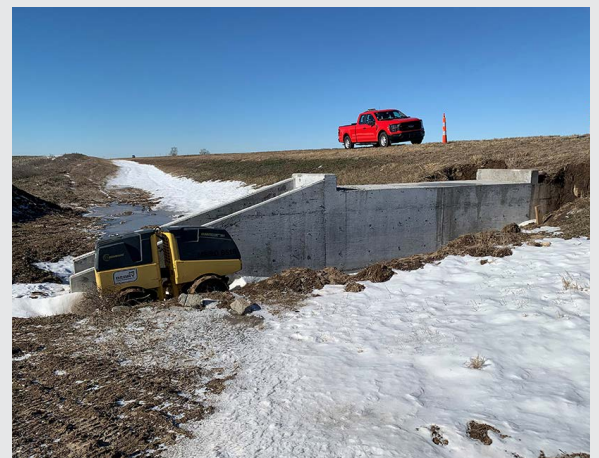
Preliminary work, as of mid-January, on the U.S. 54 passing lane project west of Mullinville. Photo by Doug Coates, Pratt
