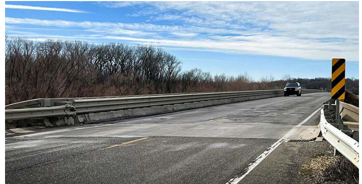
The Neosho River bridge on U.S. 59 south of Erie has undergone many deck repairs in recent years. The bridge was closed to traffic on Jan. 30. The new bridge will be completed early next year. Photo by Priscilla Petersen
