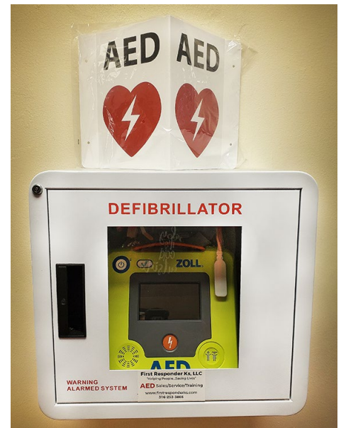
A new AED is installed in the Area Five building in Wichita. Photo by Tracy Statton.
