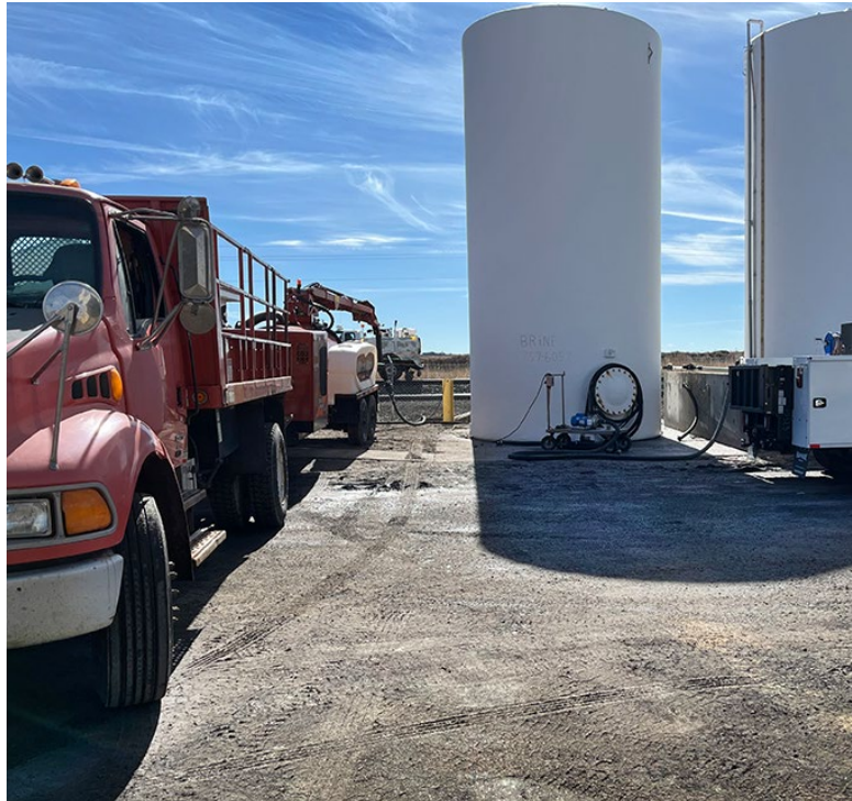
The Garden City Subarea crew worked together to contain brine that was spilled from this tank. Photo by Hector Terrones, Garden City
