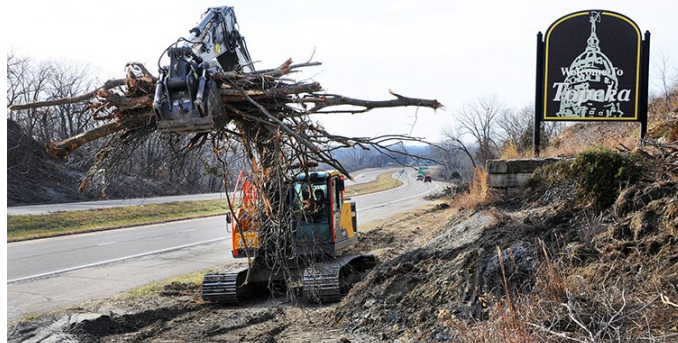
Trees are removed along U.S. 24 to prepare for upcoming work on the project.
