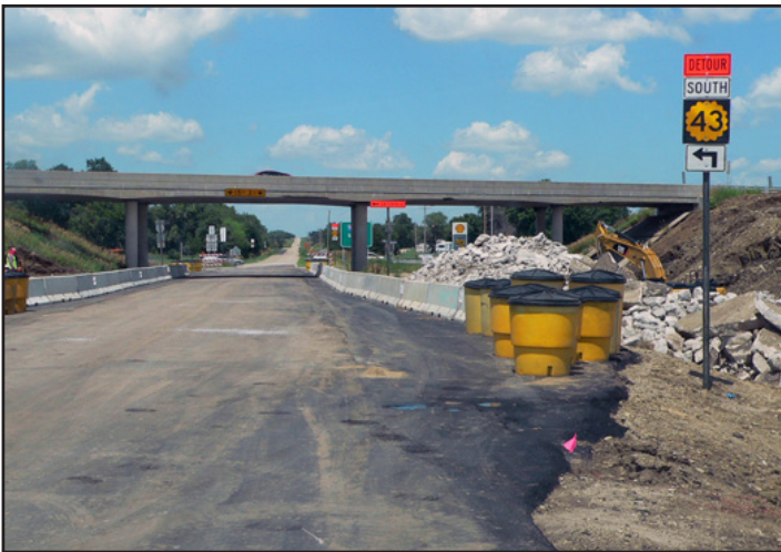
Work to remove the remains of the eastbound I-70 bridge continues at the K-43 junction.
