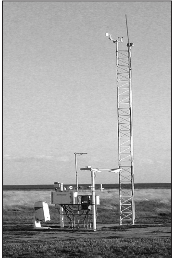
An AWOS system helps collect critical weather-related data.
