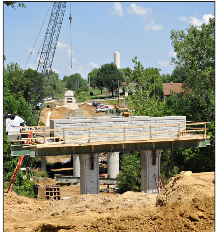
Work on the 118th Street Bridge over I-70 in Wyandotte County continues this summer. Aaron Frits' road squad and Chris Meyer's bridge squad designed the project.
