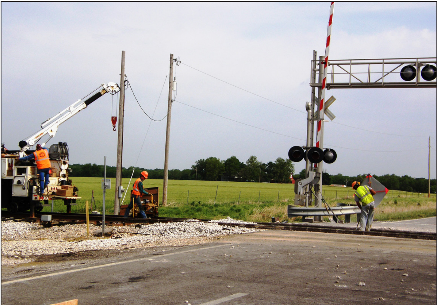
Crews with the South Kansas & Oklahoma (SKOL) Railroad replace tracks at the crossing on U.S. 169 southwest of Cherryvale. KDOT closed the highway at the crossing May 19-22 for the project.
